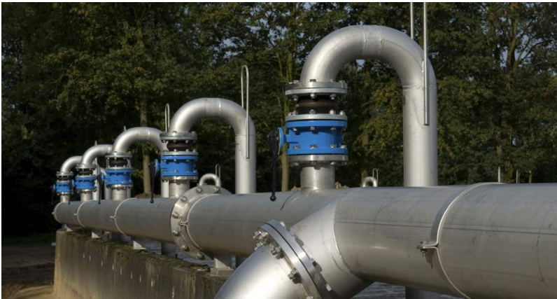
Glendora's water is supplied, in part, by the Covina Irrigation Company
