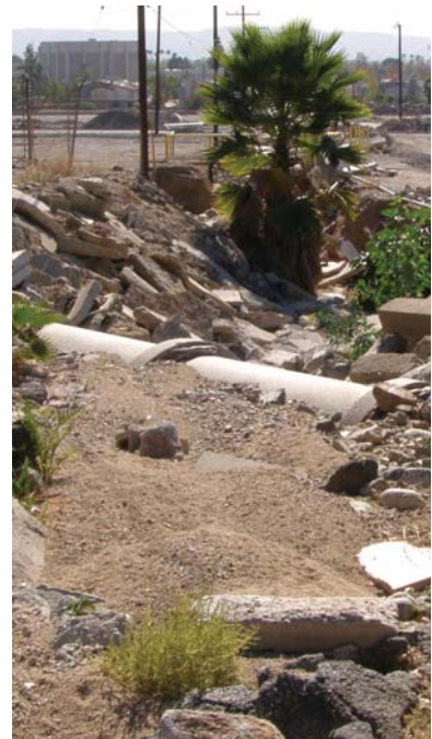
The Covina Canal partially is exposed at the southern end of Baldy Vista Creek.
